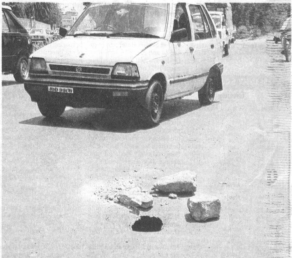
RAWALPINDI: Someone has placed stones around a hole on Liaquat Road near Tehsil Municipal Administration Office to warn motorists and pedestrians. — Sardar Heera
